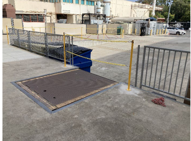
Chains / Railing Replaced After Use
