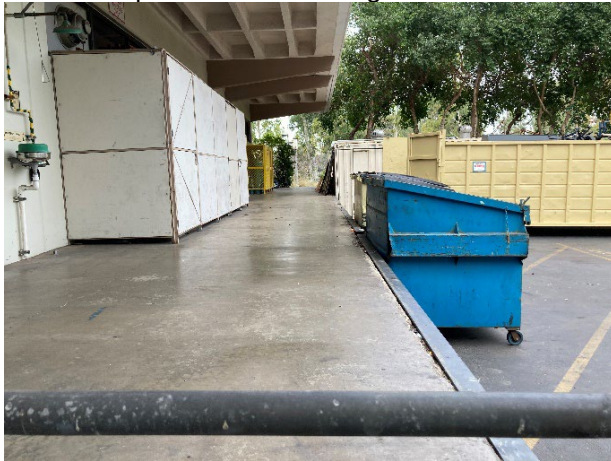
Trash Dumpster Without Railing
