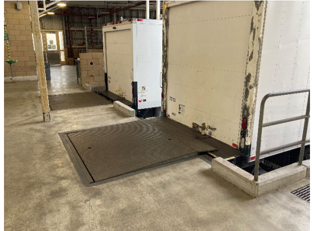
Loading Dock Leveler in Use
